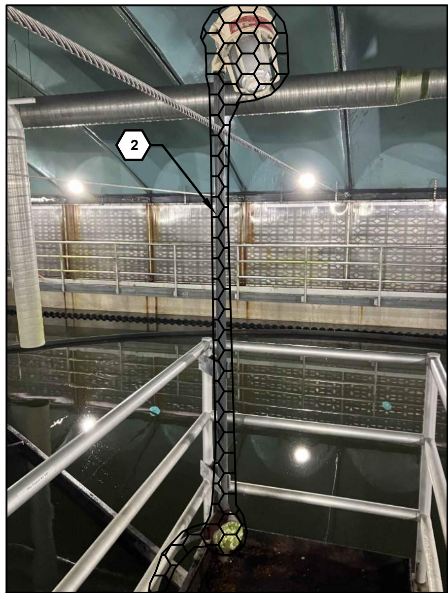
3 SECONDARY CLARIFIER NO 1 E-03 LIGHTING MAST
