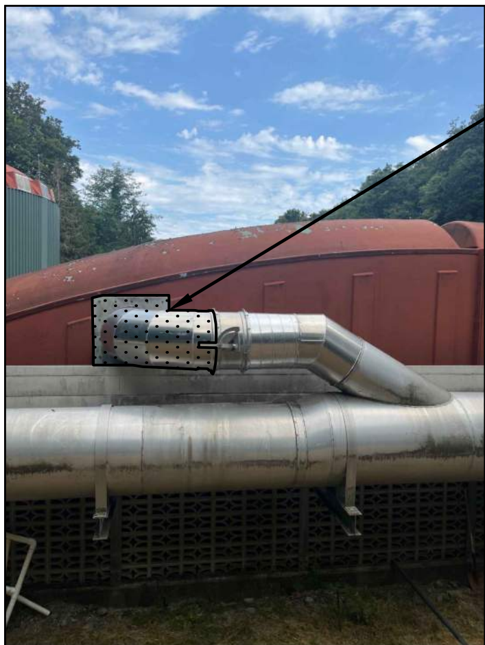
5 M-01 PRIMARY CLARIFIER #1 FOUL AIR CONNECTION
