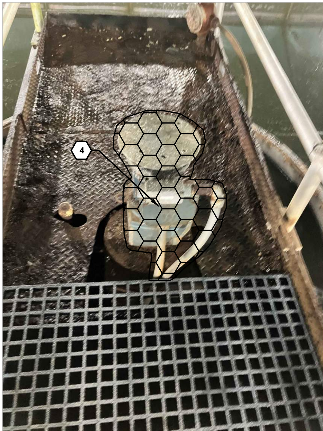
6 SECONDARY CLARIFIER NO 2 E-03 SCRAPER MOTOR
