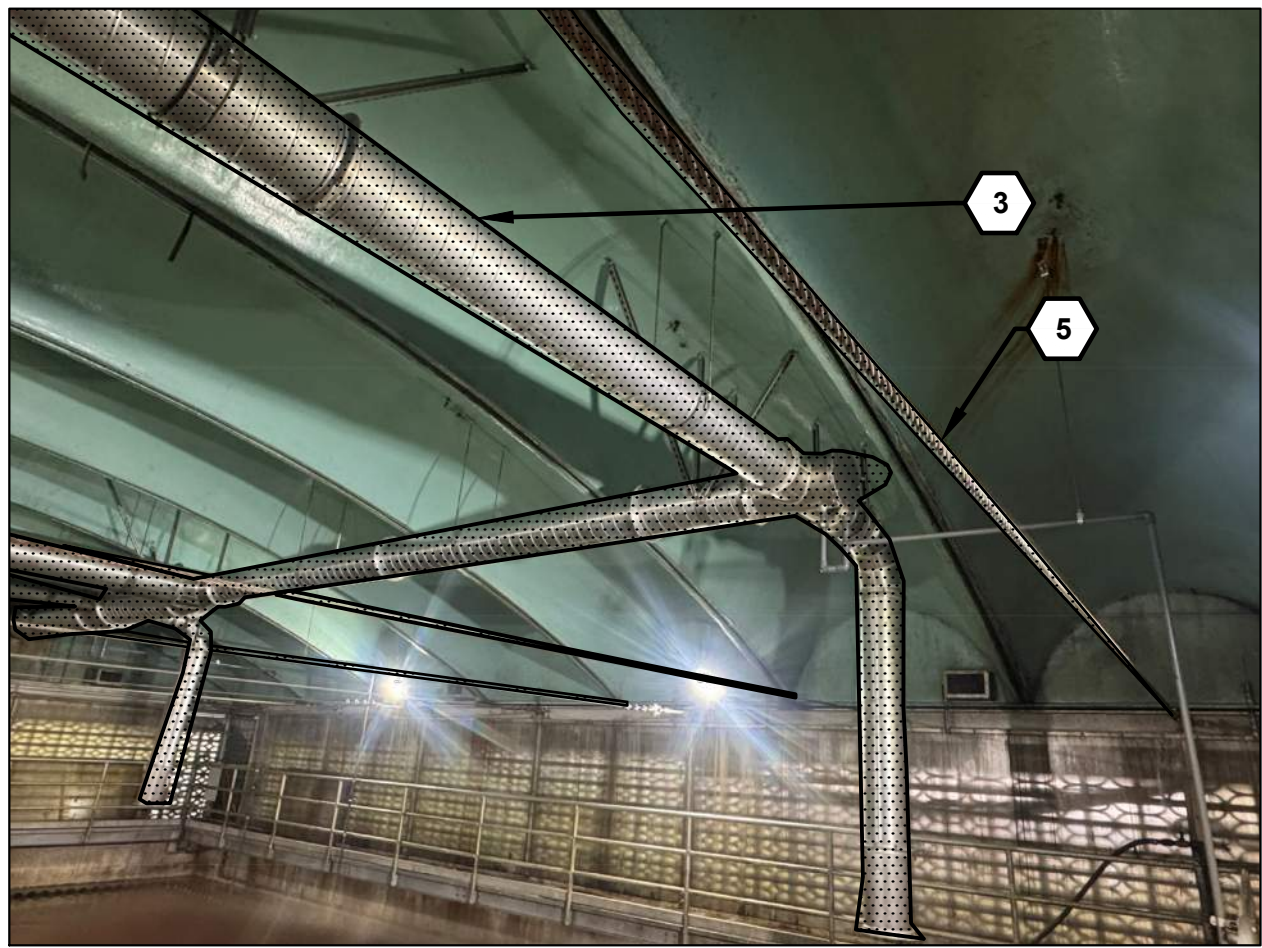
2 M-01 PRIMARY CLARIFIER FOUL AIR DUCTING
