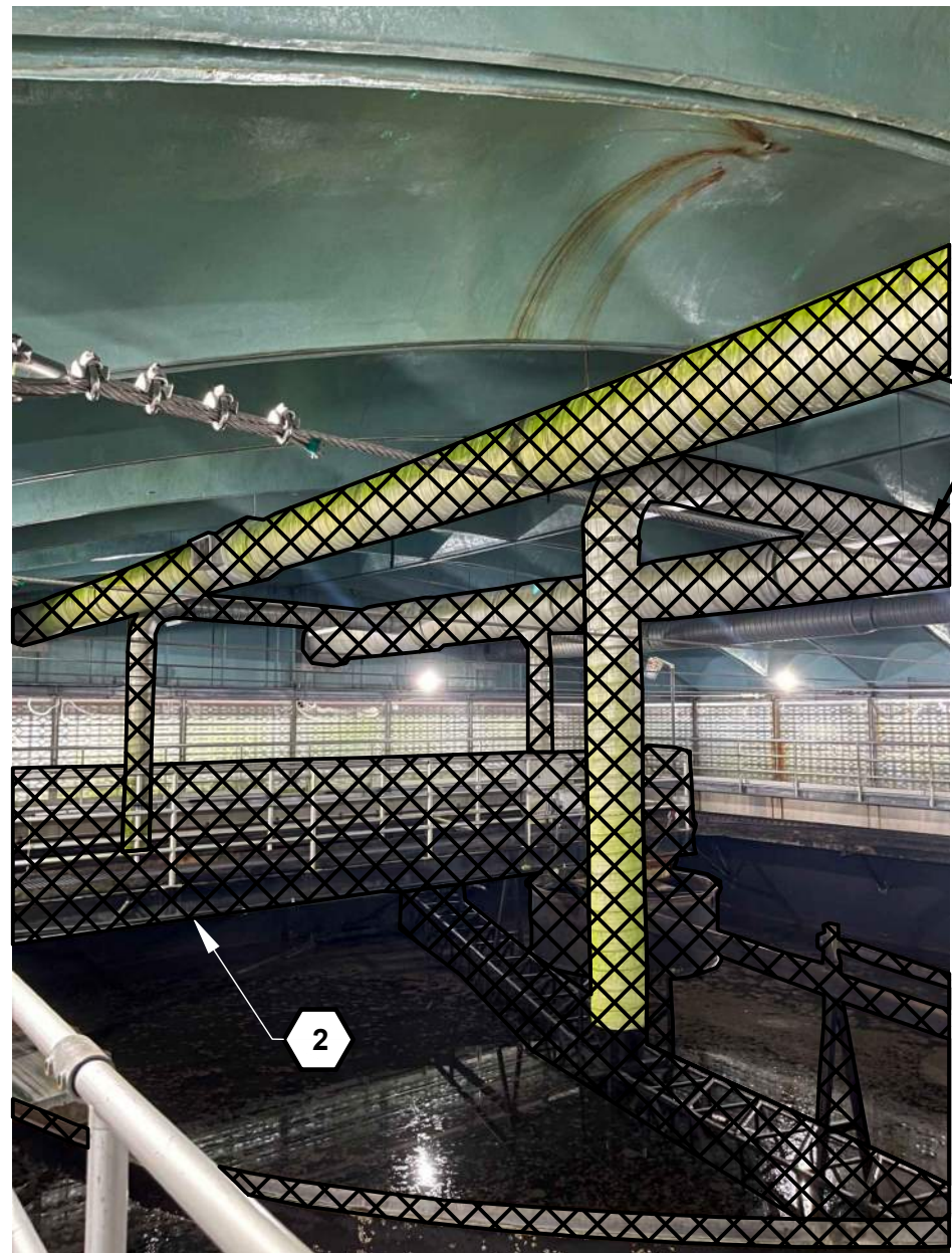
1 SECONDARY CLARIFIER D-04 FOUL AIR DUCTING (TYP)
