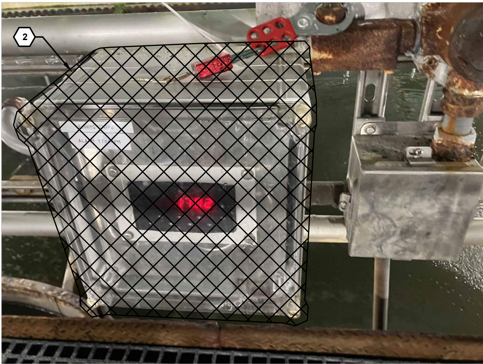
5 SECONDARY CLARIFIER NO 2 DE-02 TACHOMETER DISPLAY
