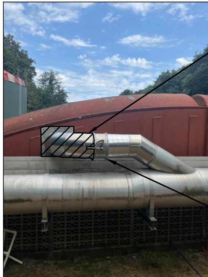
5 D-01 PRIMARY CLARIFIER #1 FOUL AIR HEADER CONNECTION
