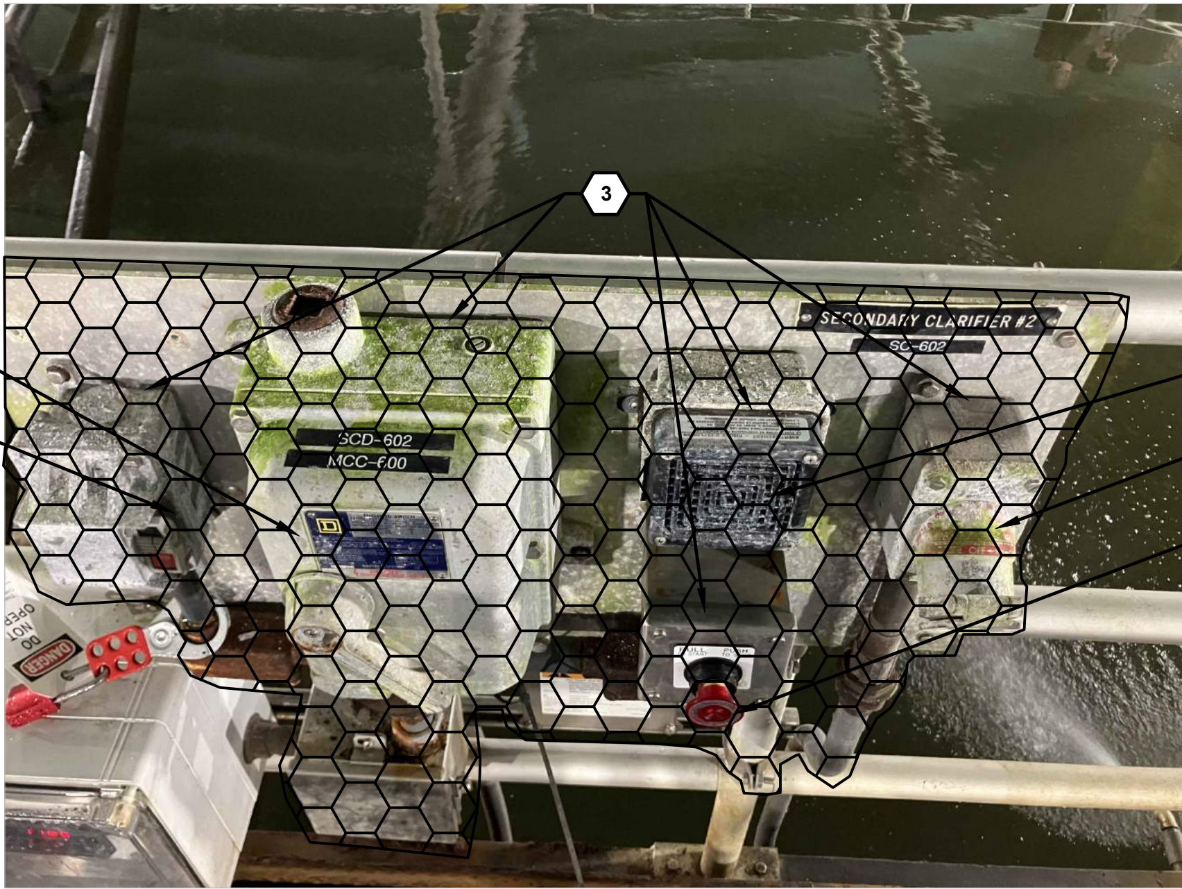
5 SECONDARY CLARIFIER NO 2 E-03 PLATFORM DEVICES
