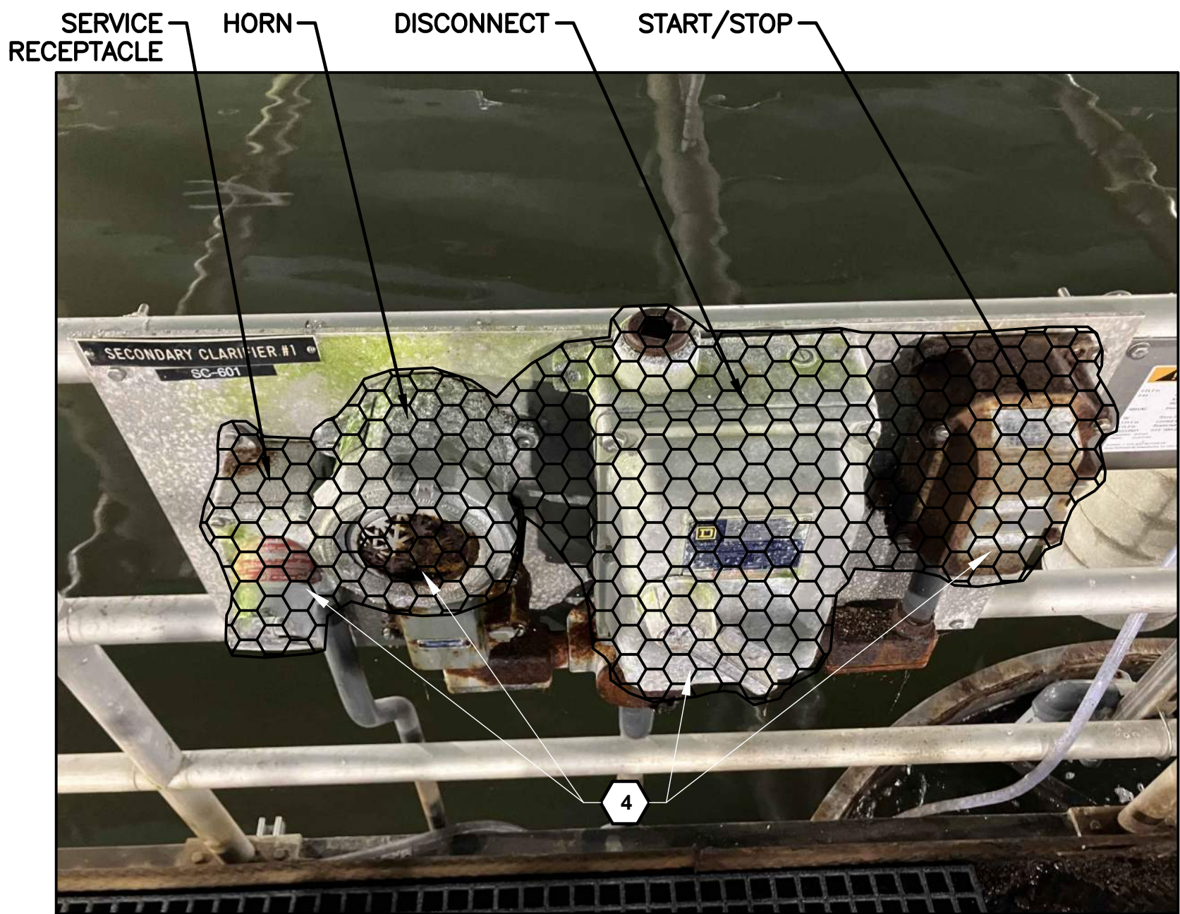
1 SECONDARY CLARIFIER NO 1 E-03 PLATFORM DEVICES
