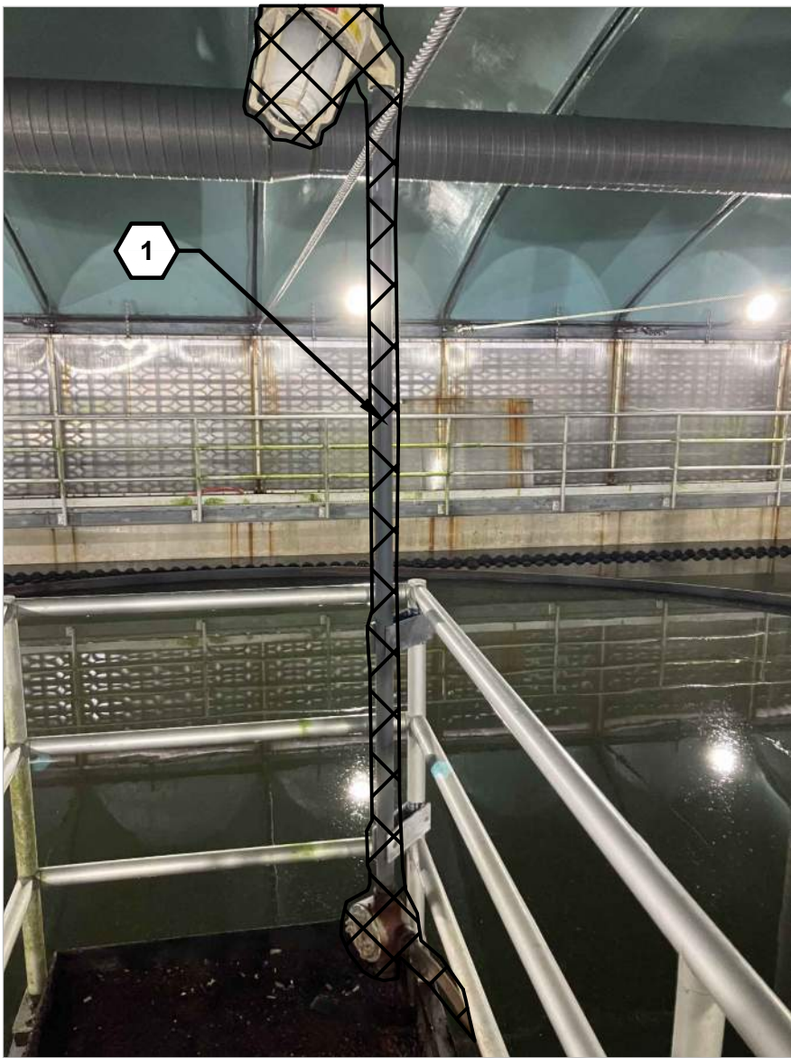
4 SECONDARY CLARIFIER NO 2 DE-02 LIGHTING MAST
