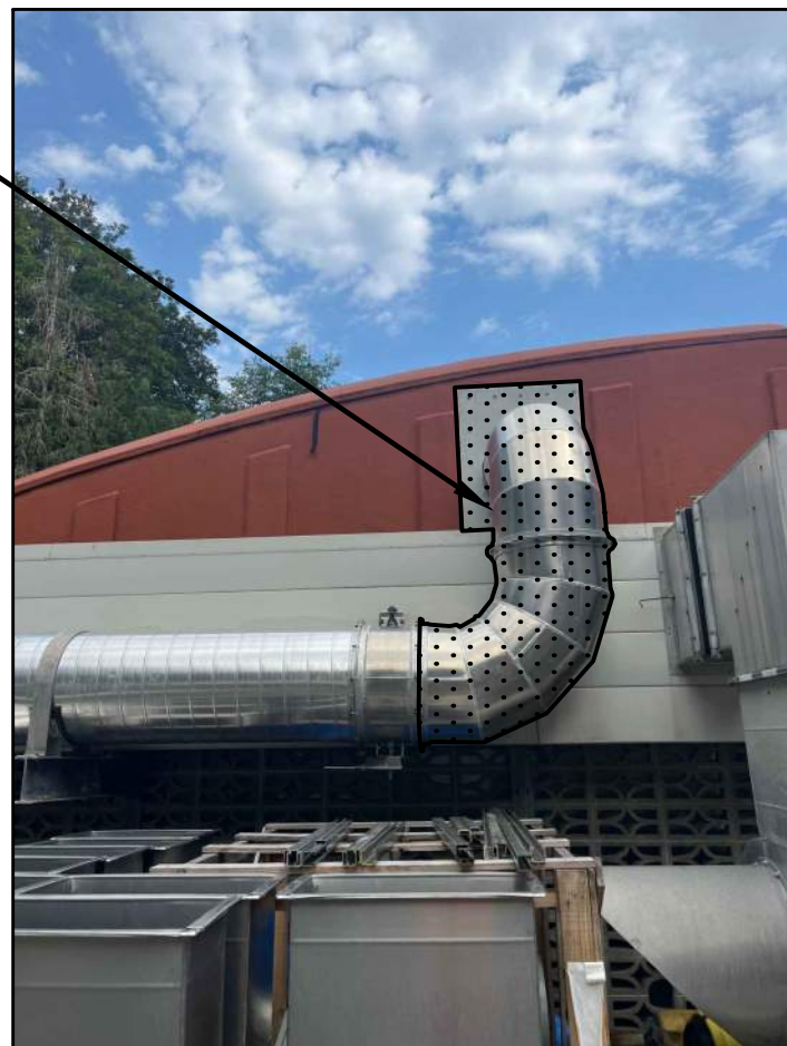
6 M-01 PRIMARY CLARIFIER #2 FOUL AIR CONNECTION
