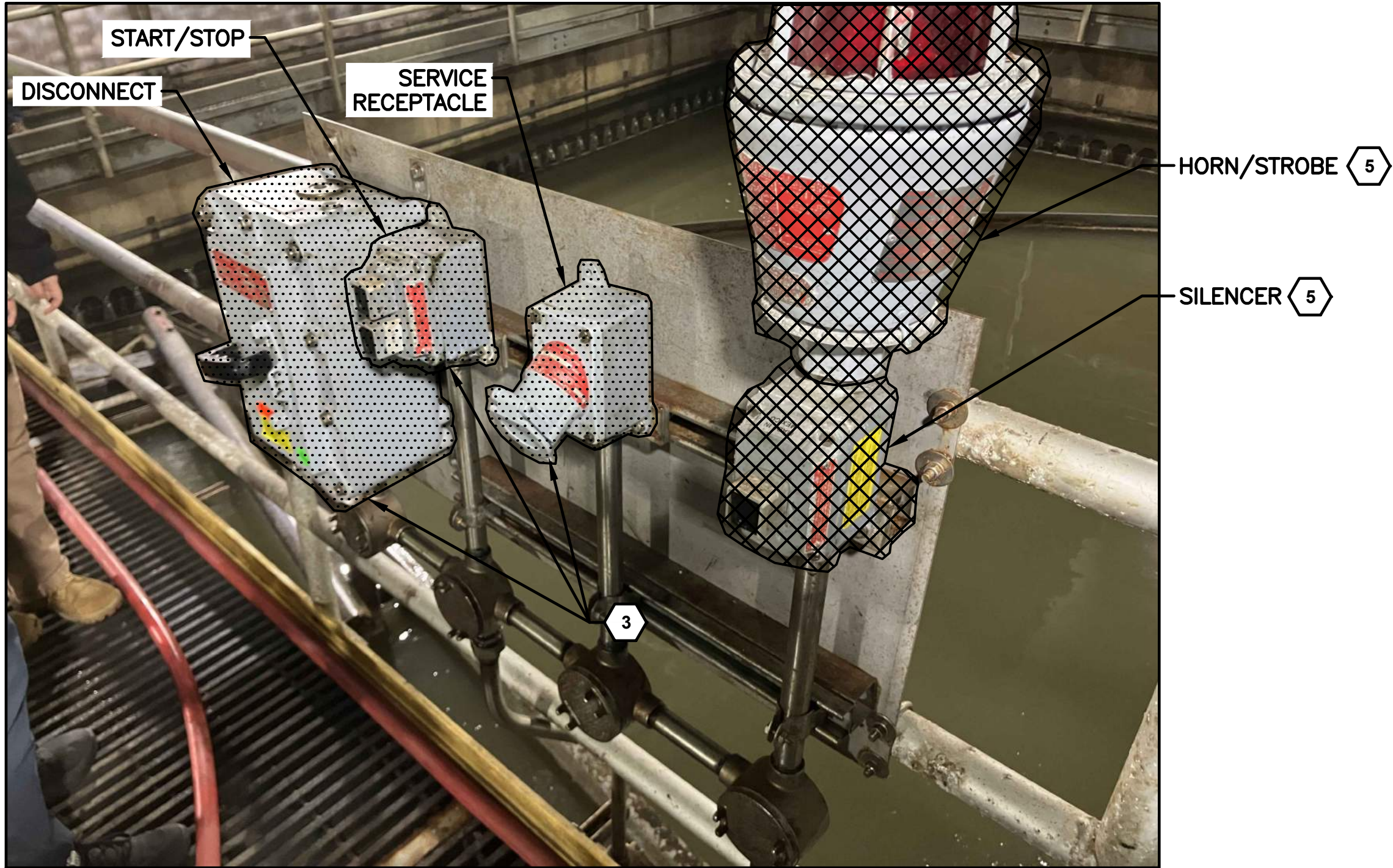
1 PRIMARY CLARIFIER NO 1 E-02 PLATFORM DEVICES
