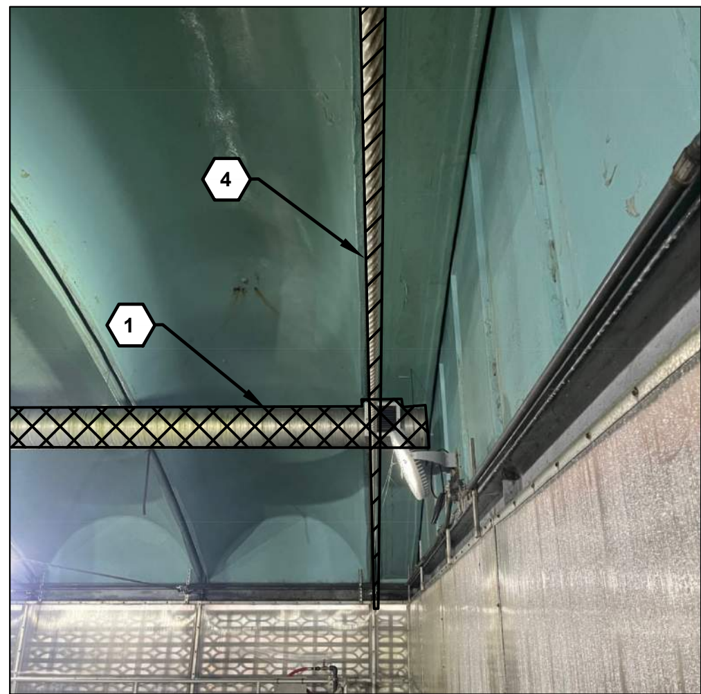
6 SECONDARY CLARIFIER D-04 FOUL AIR DUCTING (TYP)
