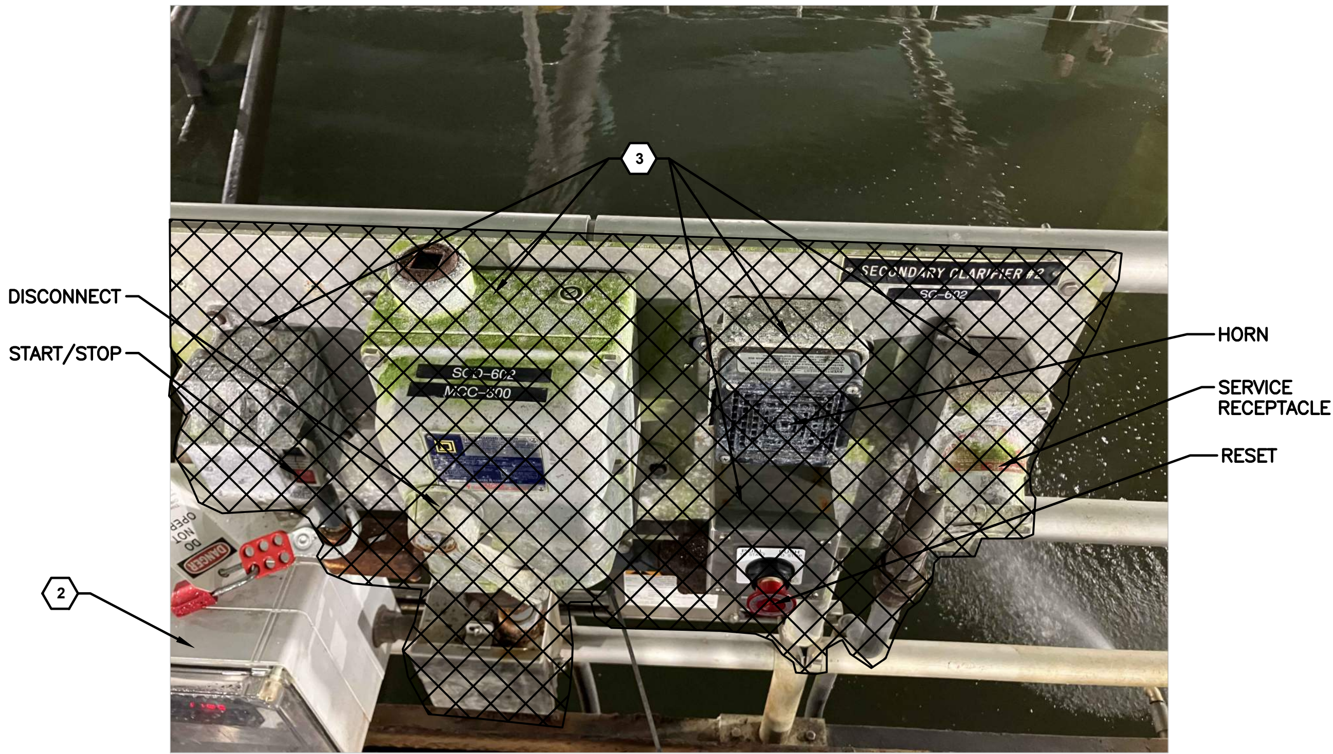
6 SECONDARY CLARIFIER NO 2 DE-02 PLATFORM DEVICES
