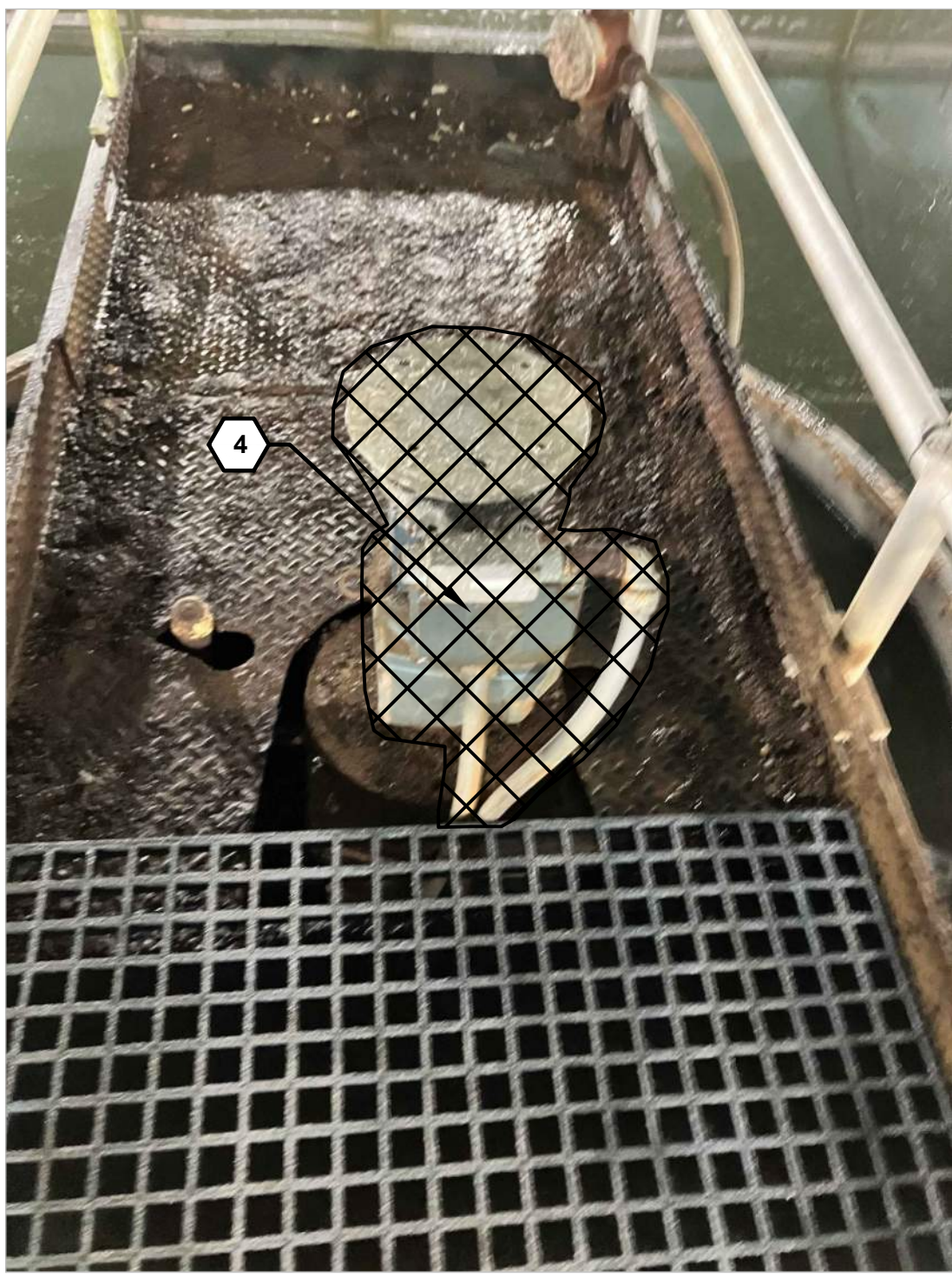
7 SECONDARY CLARIFIER NO 2 DE-02 SCRAPER MOTOR
