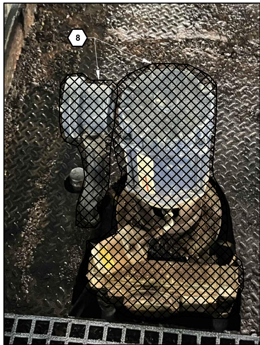
2 SECONDARY CLARIFIER NO 1 DE-02 SCRAPER MOTOR
