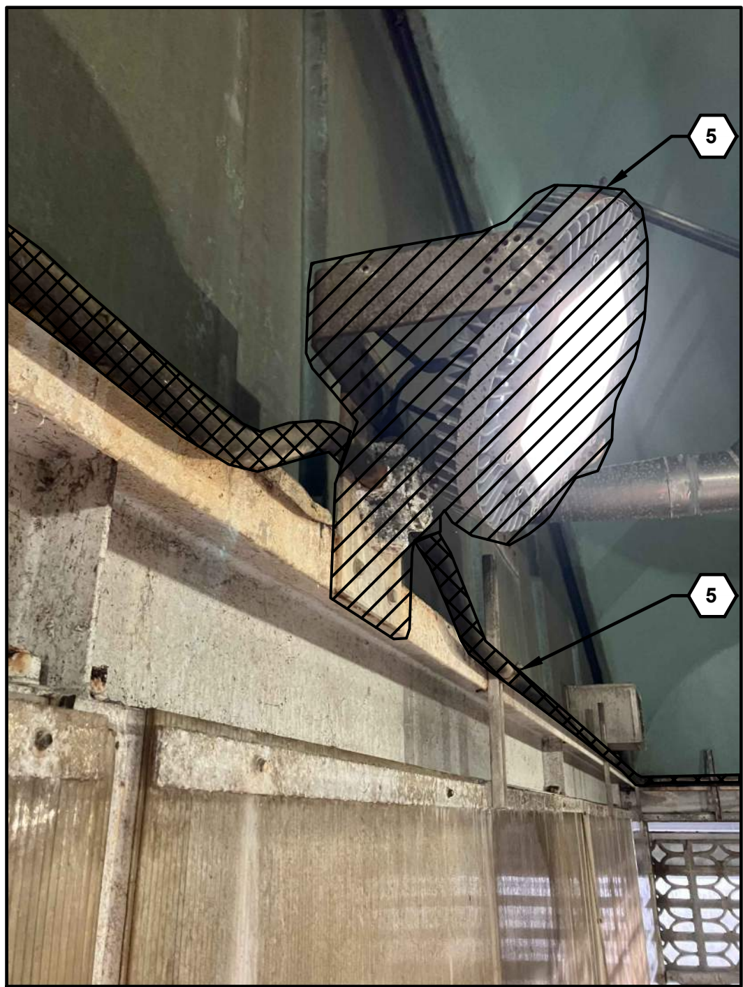
5 PRIMARY CLARIFIER DE-01 PERIMETER LUMINAIRES
