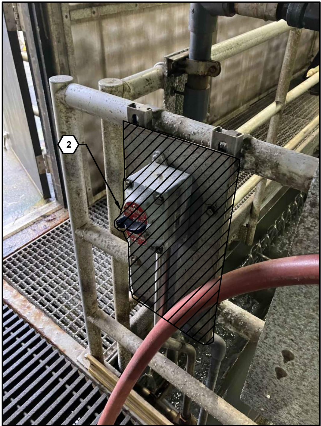
4 PRIMARY CLARIFIER NO 1 DE-01 PLATFORM WALKWAY LIGHT SWITCH
