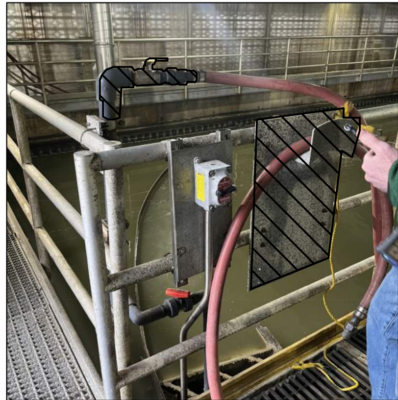
1 D-02 PRIMARY CLARIFIER PROCESS WATER WASHDOWN STATION
