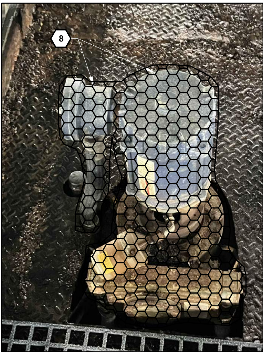
2 SECONDARY CLARIFIER NO 1 E-03 SCRAPER MOTOR
