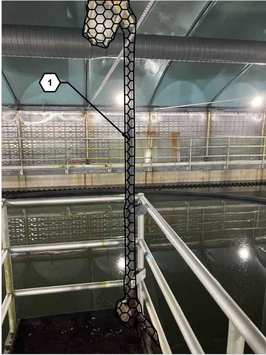
4 SECONDARY CLARIFIER NO 2 E-03 LIGHTING MAST
