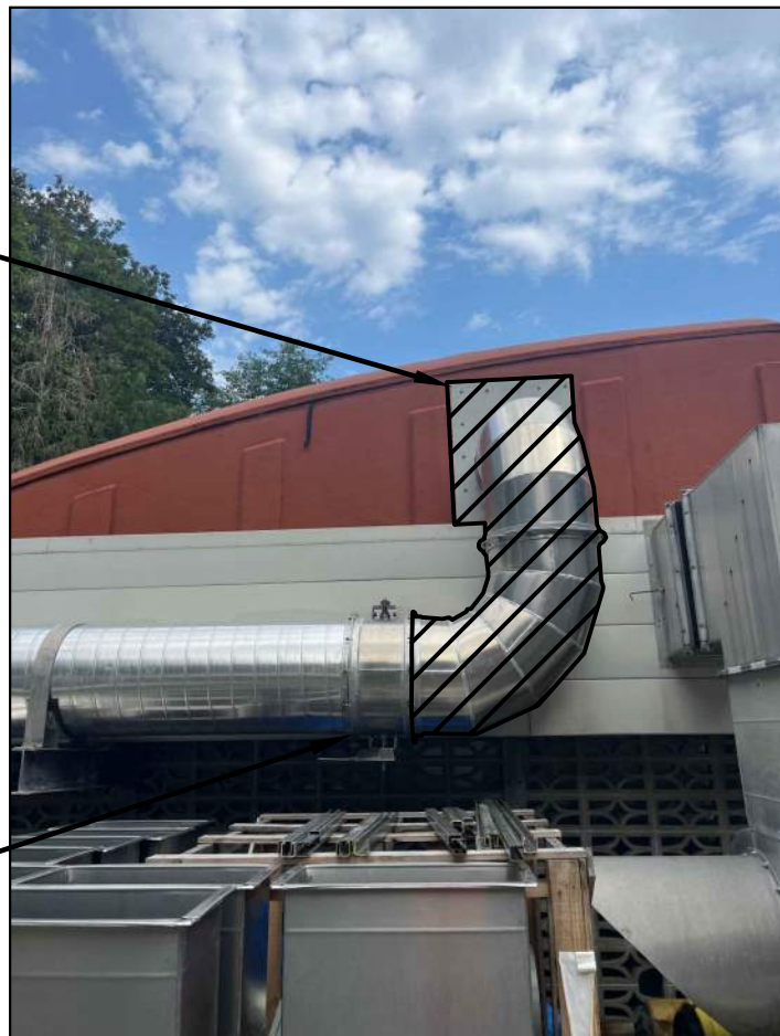
6 D-01 PRIMARY CLARIFIER #2 FOUL AIR HEADER CONNECTION
