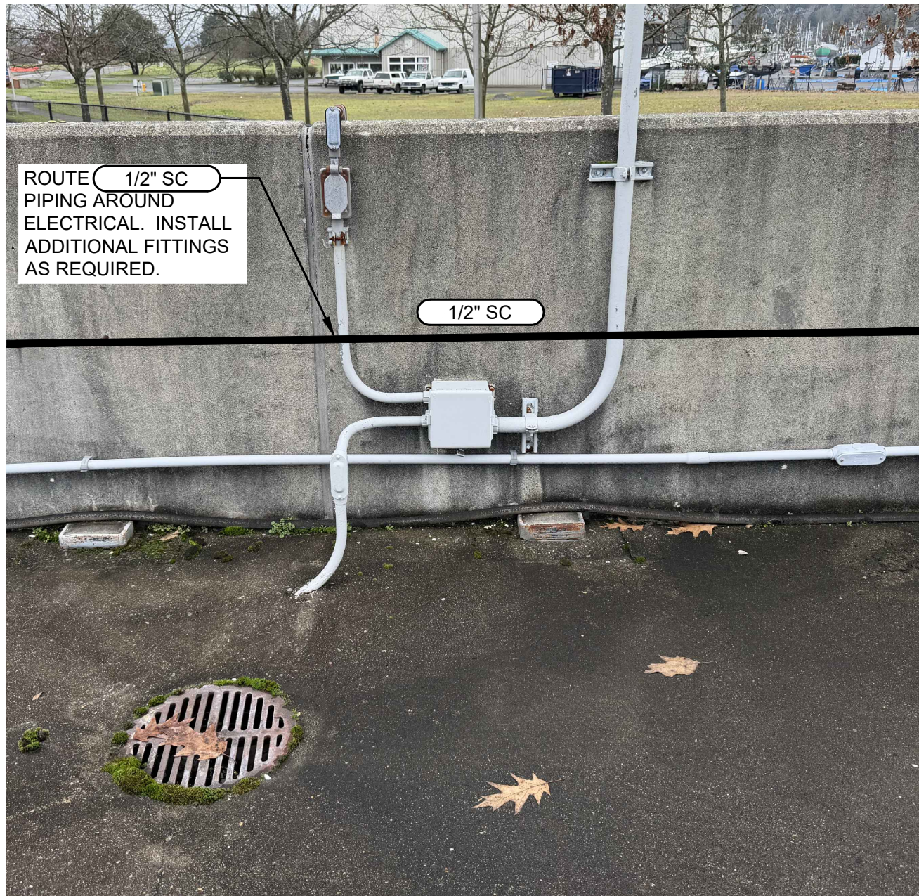
PHOTO 5 SUPPLEMENTAL CARBON PIPE ROUTING
