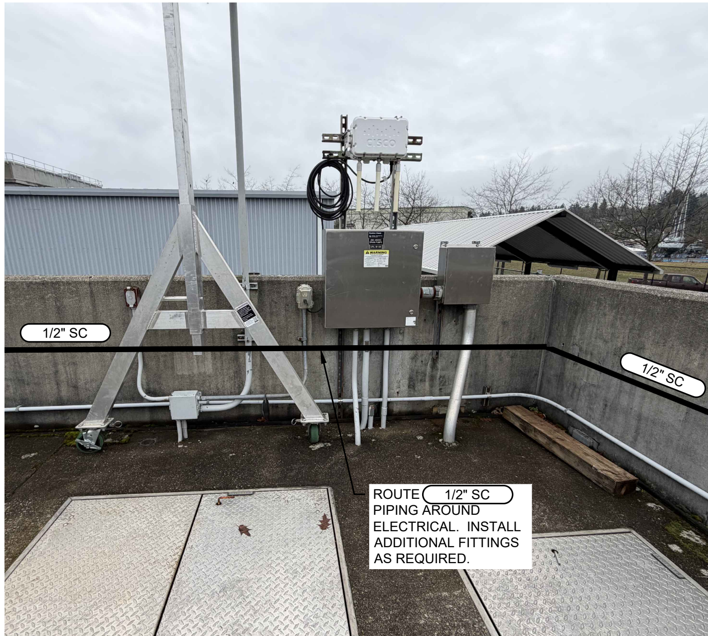
PHOTO 4 SUPPLEMENTAL CARBON PIPE ROUTING
