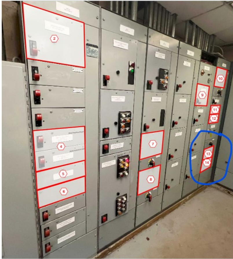
PHOTO DETAIL 1 MCC-I SECTIONS 8-13
