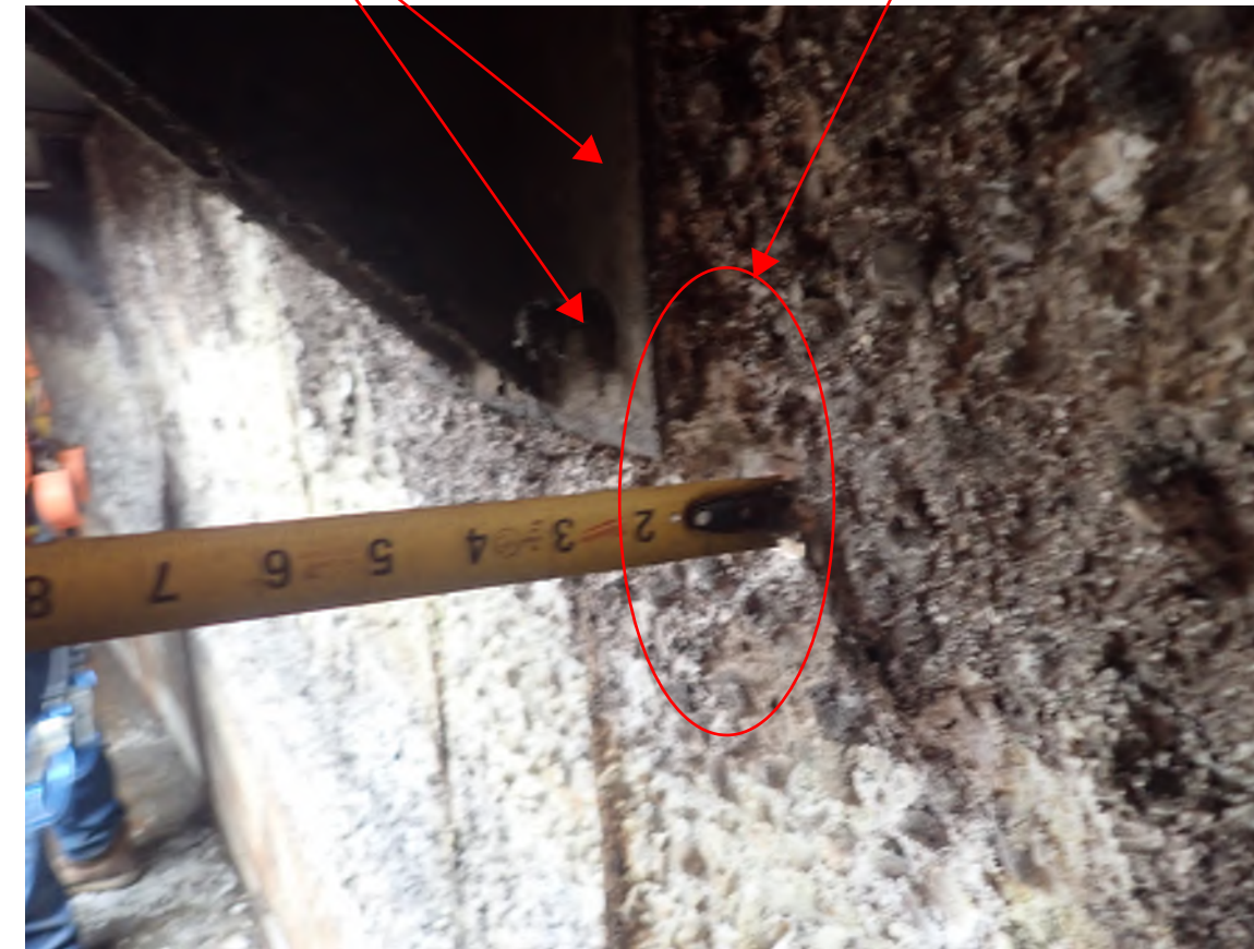
COMPROMISED CONCRETE BEHIND (E) SUPPORT BRACKET
