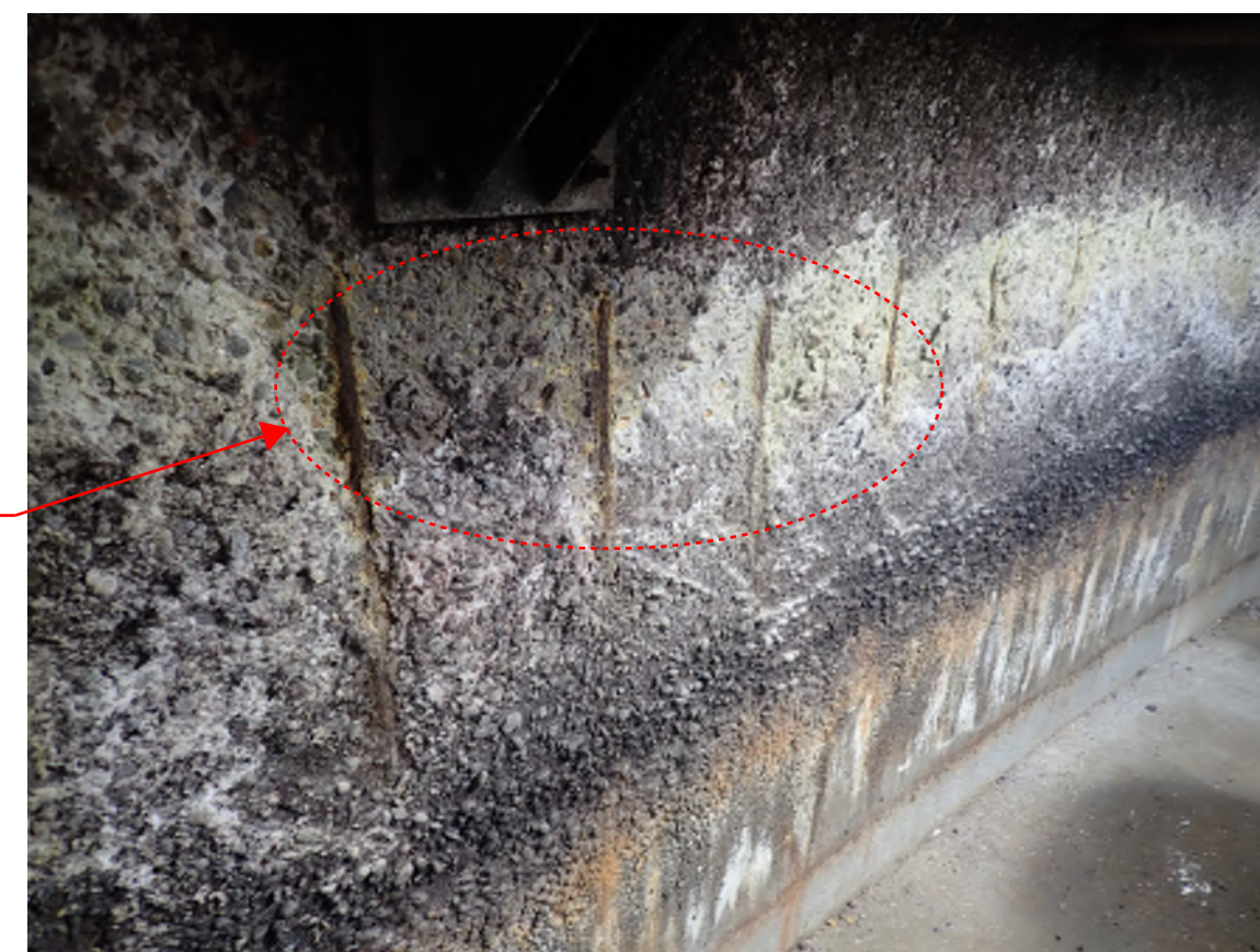
EXPOSED AND CORRODED REBAR & COMPROMISED CONCRETE
