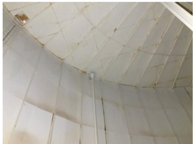
Interior upper shell and view of overhead. Note Vertical stiffeners placed 66" on center.
