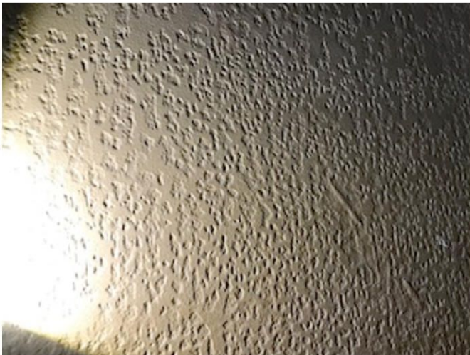
Large concentration of existing pitted steel at An area of the shell wall. Coating appears sound However and actively protecting the steel.
