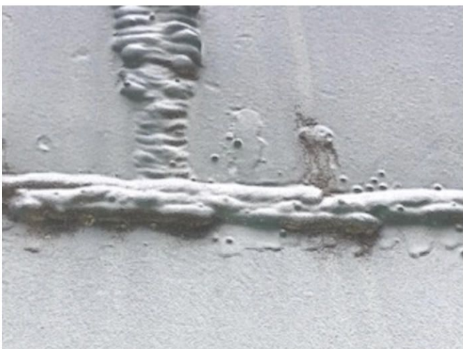
Weld globules and spatter typical at exterior welds.
