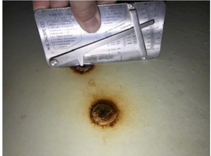
Depth measurement of localized pitting at floor. Depth ranged from 1/8 th to 3/16 th .
