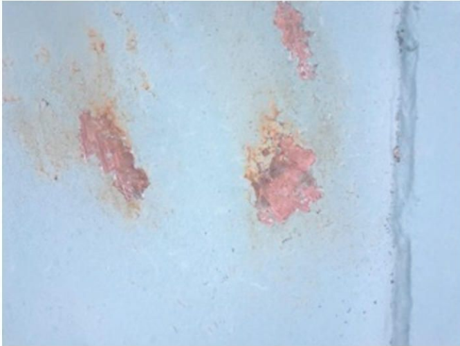
Area at exterior roof where coating sample was removed for heavy metals testing at lab.
