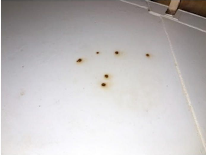
Localized pitting/corrosion cells observed at floor plates within the interior.
