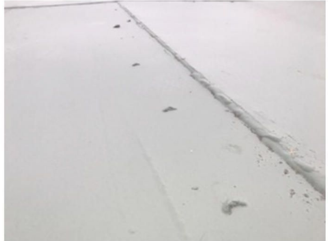
Residual weld scabs and weld spatter observed at numerous locations of the exterior roof/shell.
