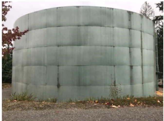
Exterior – East quad shows obvious “ripples” at The exterior rings from possible shifting possibly caused during Nisqually earthquake.
