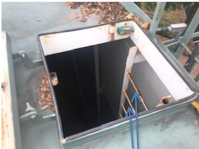
Exterior roof hatch, poor condition of coatings at Interior ladder assembly.
