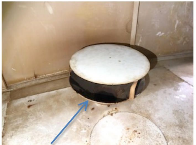
Floor drain and area at floor where interior sample was recovered for lab analysis.
