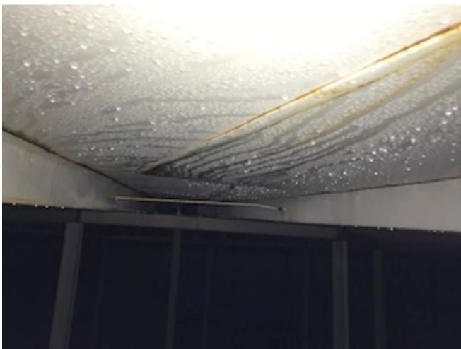
Interior overhead depicting the plate overlaps w/ Crevice corrosion and rust bleed.
