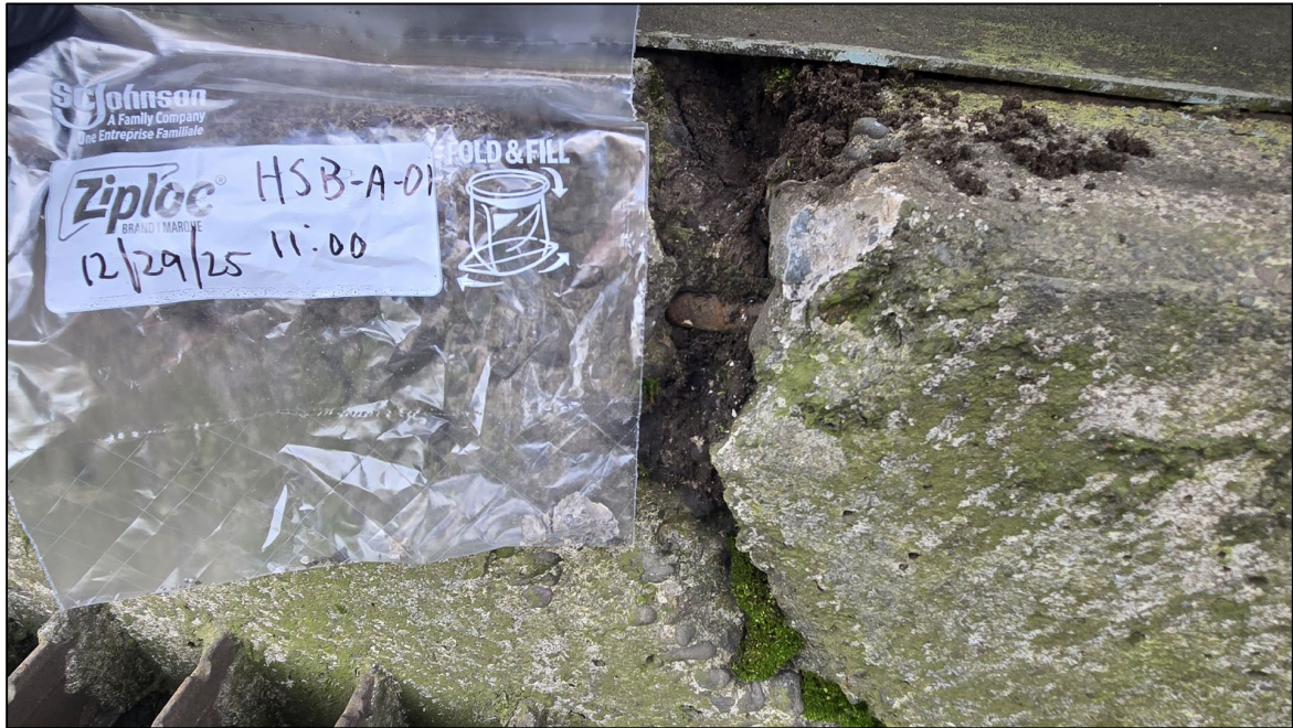
Photograph 3. Concrete sample HSB-A-01 collected from the west end of the south curb of the Heron Street Bridge.
