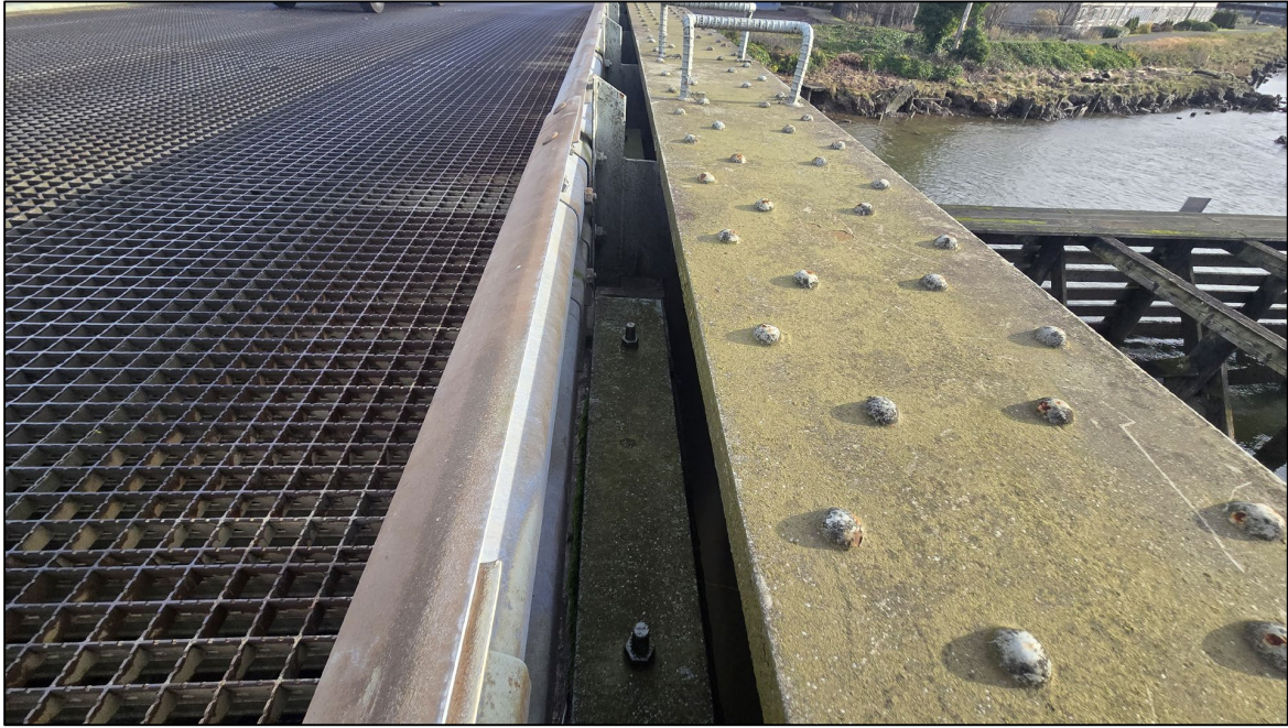
Photograph 5. Weight blocks bolted to the south curb near the middle of the Heron Street Bridge.
