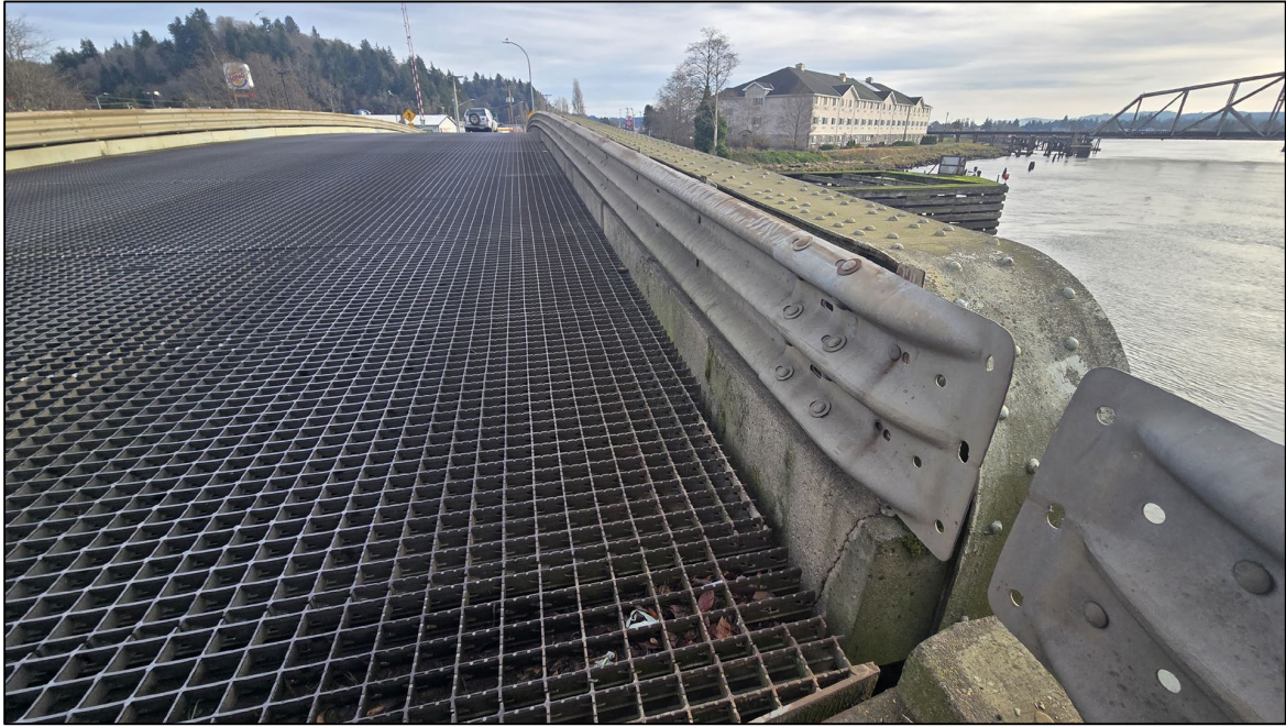
Photograph 1. Looking east along the south curb of the US-12 Heron Street Bridge.
