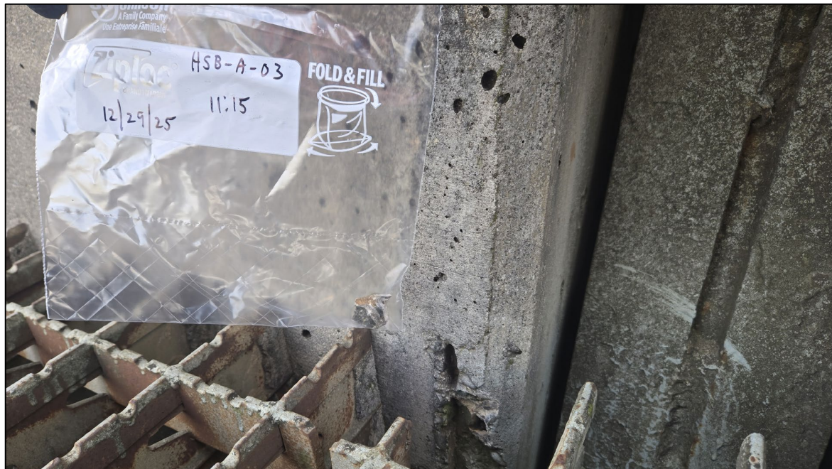
Photograph 4. Concrete sample HSB-A-03 collected from the east end of the south curb of the Heron Street Bridge .
