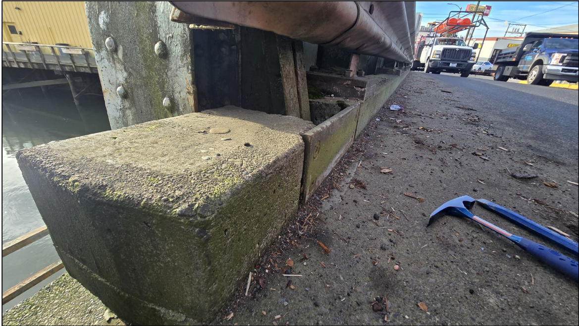
Photograph 9. East end of the approach to the deck of the Heron Street Bridge.
