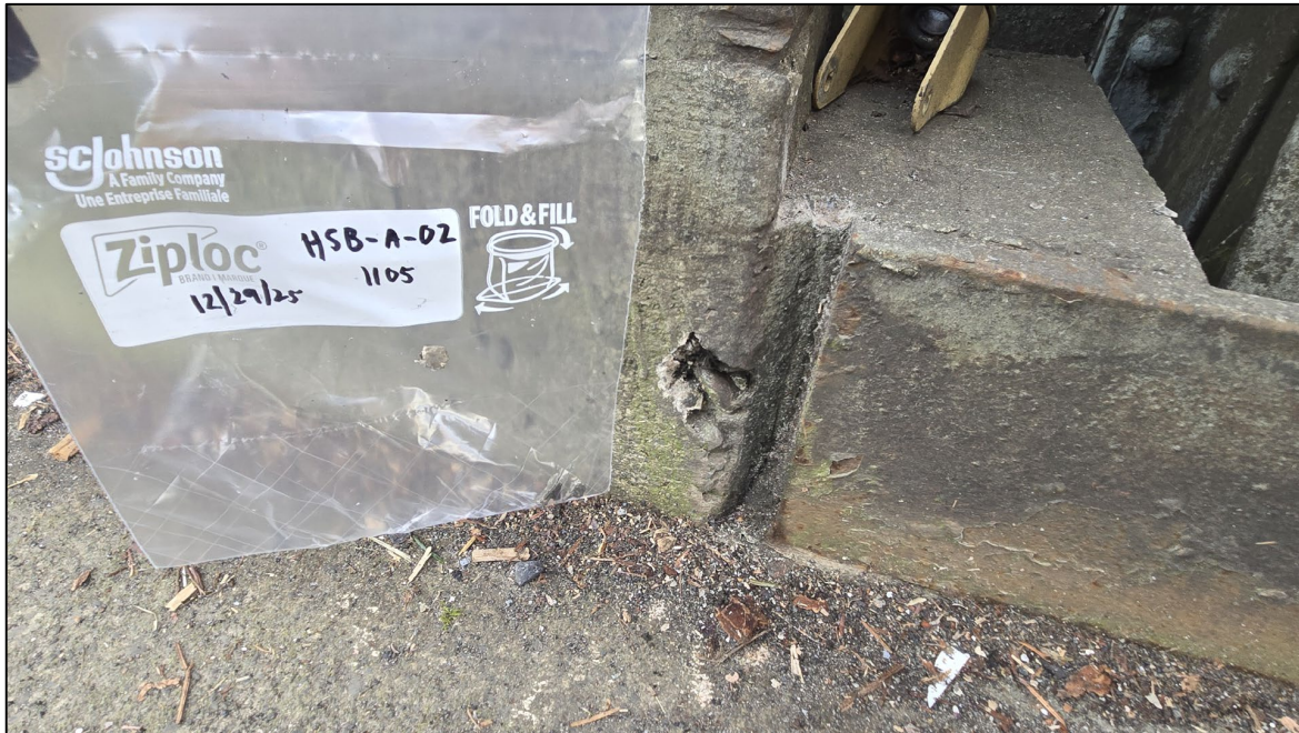
Photograph 8. Concrete sample HSB-A-02 collected from the west end of the south curb of the approach to the Heron Street Bridge deck.
