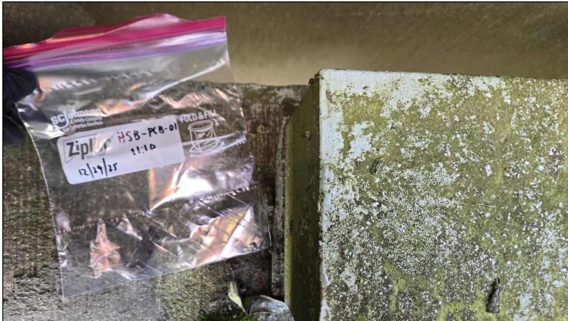
Photograph 6. Gasket material sample HSB-PCB-01 collected from the gasket between the south curb and weight blocks near the middle of the Heron Street Bridge deck.
