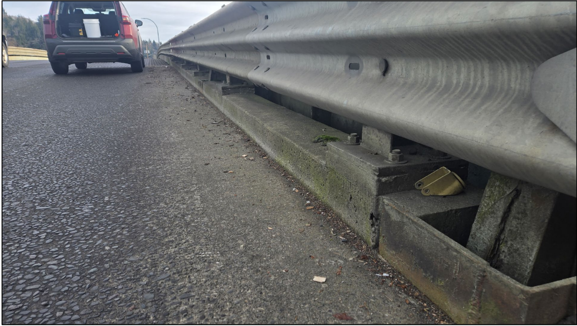
Photograph 7. Concrete curb on the approach to the deck of the Heron Street Bridge.
