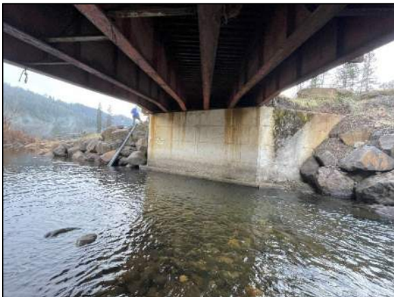
Photograph 3. Site photograph taken from underneath the bridge, looking north toward the northern abutment.
