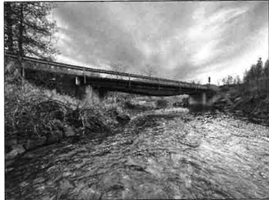
Photograph 2. Site photograph taken from upstream of the bridge, looking east toward the bridge.
