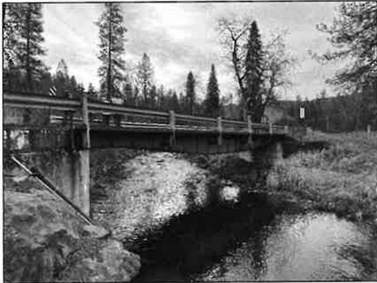
Photograph 1. Site photograph taken from downstream of the bridge, looking east toward the bridge.
