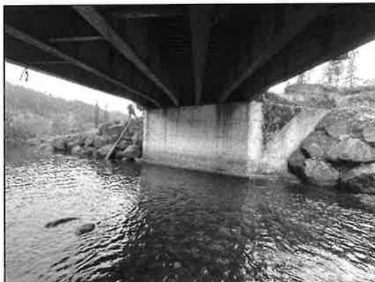
Photograph 3. Site photograph taken from underneath the bridge, looking north toward the northern abutment.
