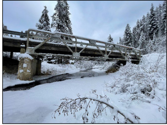
Photograph 2. Site photograph taken from downstream of the bridge, looking east toward the bridge.
