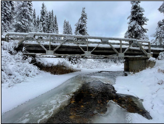
Photograph 1. Site photograph taken from upstream of the bridge, looking west toward the bridge.
