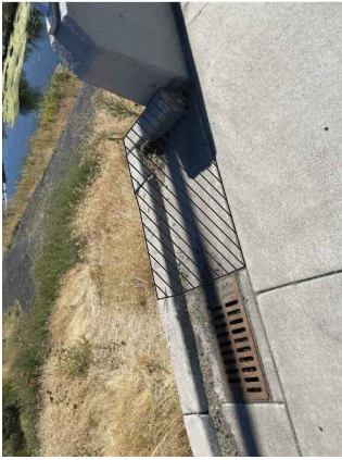
TYPICAL DAMAGED APPROACH CURB NE CORNER SHOWN
